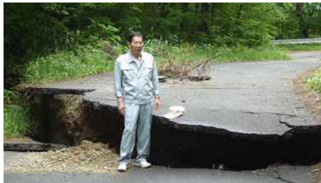
Damage to roads, picture from Kurihara City, Miyagi Prefecture.
